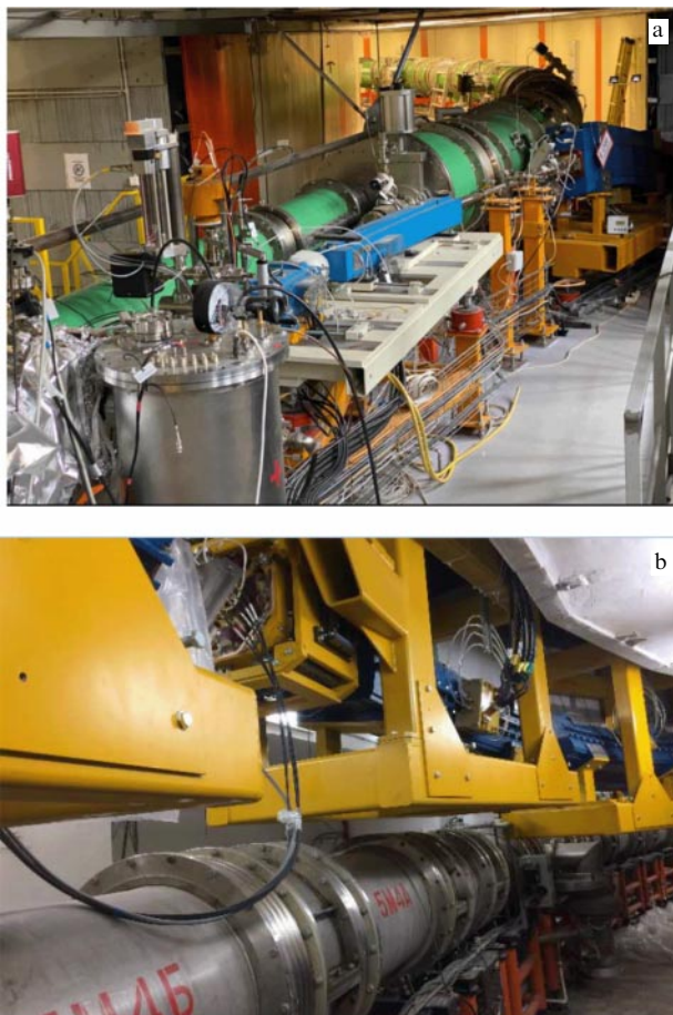
Figure 4. (a) Elements of the fast extraction system in the third straight gap. (b) Booster–Nuclotron transport channel.
